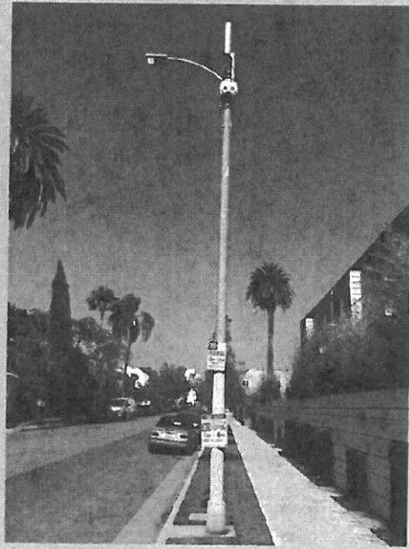
Typical placement on a street light
